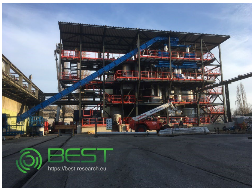
Gasification and FT demo plant under construction in Vienna at BEST – Bioenergy and Sustainable Technologies (former BIOENERGY 2020+ GmbH).
