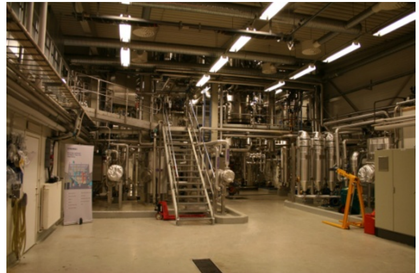
Ground floor of gasification plant
