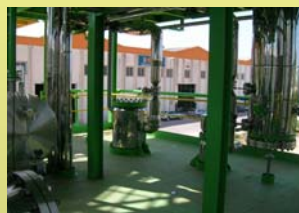
Pilot plant first level
