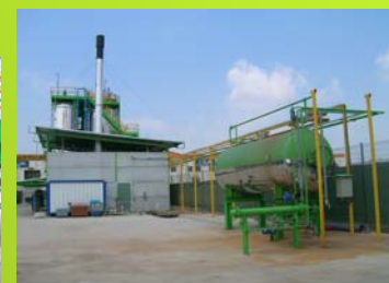
Bioethanol store tank
