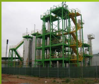
PERSEO experimental pilot plant
